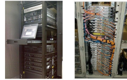
Front of a rack Rear of a rack
